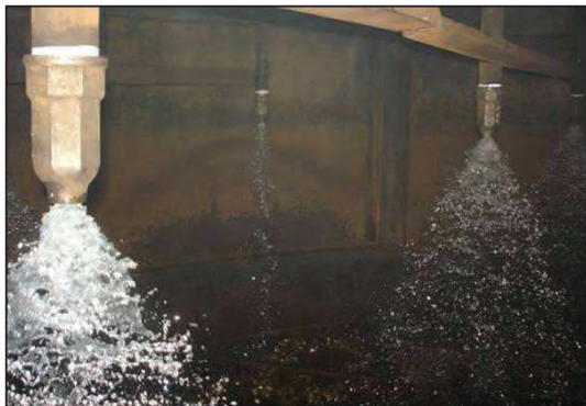
FIGURE 2. Water testing quickly identifies nozzle plugging
