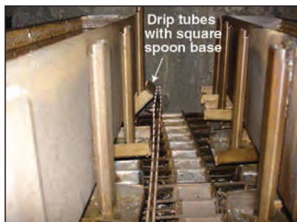
FIGURE 5. Some drip tubes were bent, causing uneven liquid distribution
