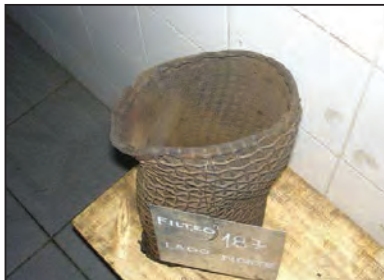
FIGURE 11. This deformed mesh taken from the Y filter would allow solids to pass to the spray nozzles and potentially cause plugging
