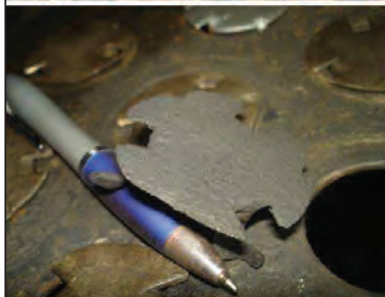
FIGURE 14A (top) and B (bottom). Some valves on the trays were found to be missing or corroded
