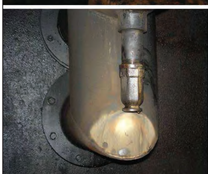
FIGURE 8A (top) and 8B (bottom). This design mistake caused a pipe to be wetted from a nozzle, which could potentially cause corrosion
