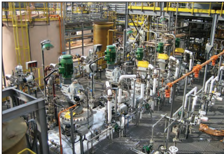
FIGURE 3. Shown here is the pressure oxidation autoclave at Vale SA's plant in the Carajás region of Brazil. The plant is the first commercial hydrometallurgical plant using CESL Ltd's technology
