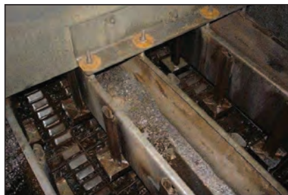
FIGURE 6. Even though dirt was found in the distributor, the design compensated for the fouling
