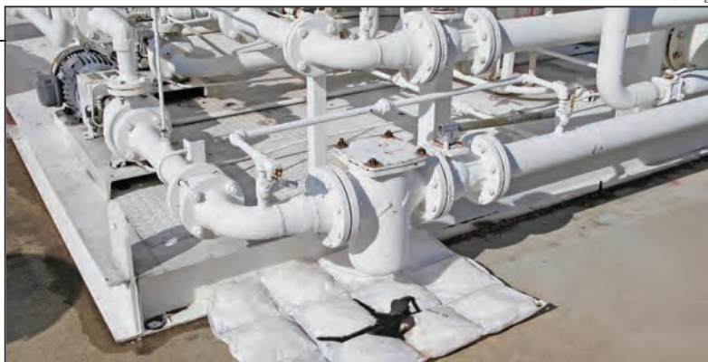
FIGURE 2. Absorbent products made from 80% recycled cellulose fibers are suitable for cleaning up most leaks, drips and spills. The cotton-based products are capable of absorbing many times more than traditional materials
