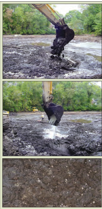
FIGURE 1. Hazardous lagoon sludge is treated with super-absorbent polymers, rendering it a solidified substance that is easier to remove from the site
