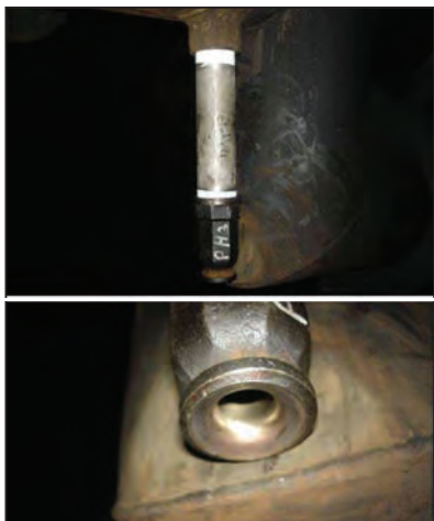
FIGURE 9A and B. A longer nozzle might have caused a worse corrosion problem to the pipe weld
