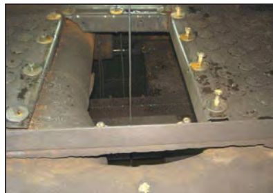
FIGURE 18. During installation of the distributors in the column, downcomers were damaged
