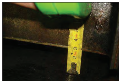
FIGURE 17. Check that downcomer clearances are within specifications
